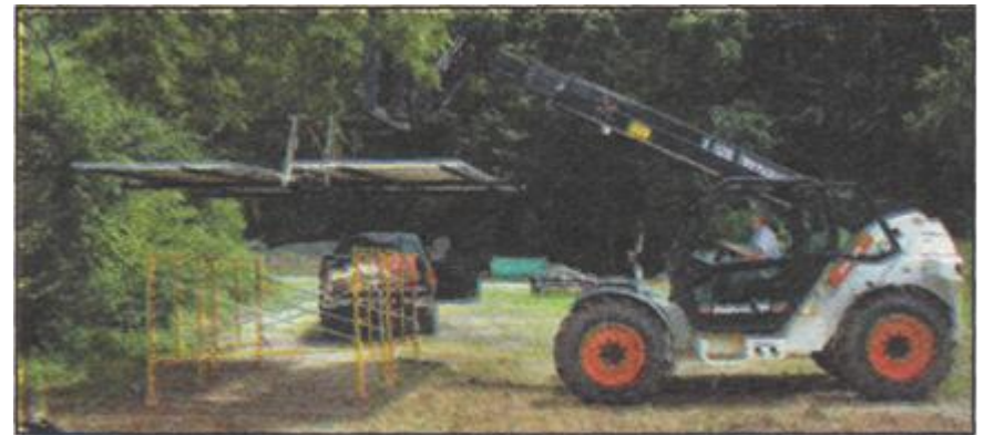
Adriann Perry uses a Bobcat to hoist solar panels for a 2-kilowatt, pole-mounted system at Codorus State Park in Hanover, Pa.
