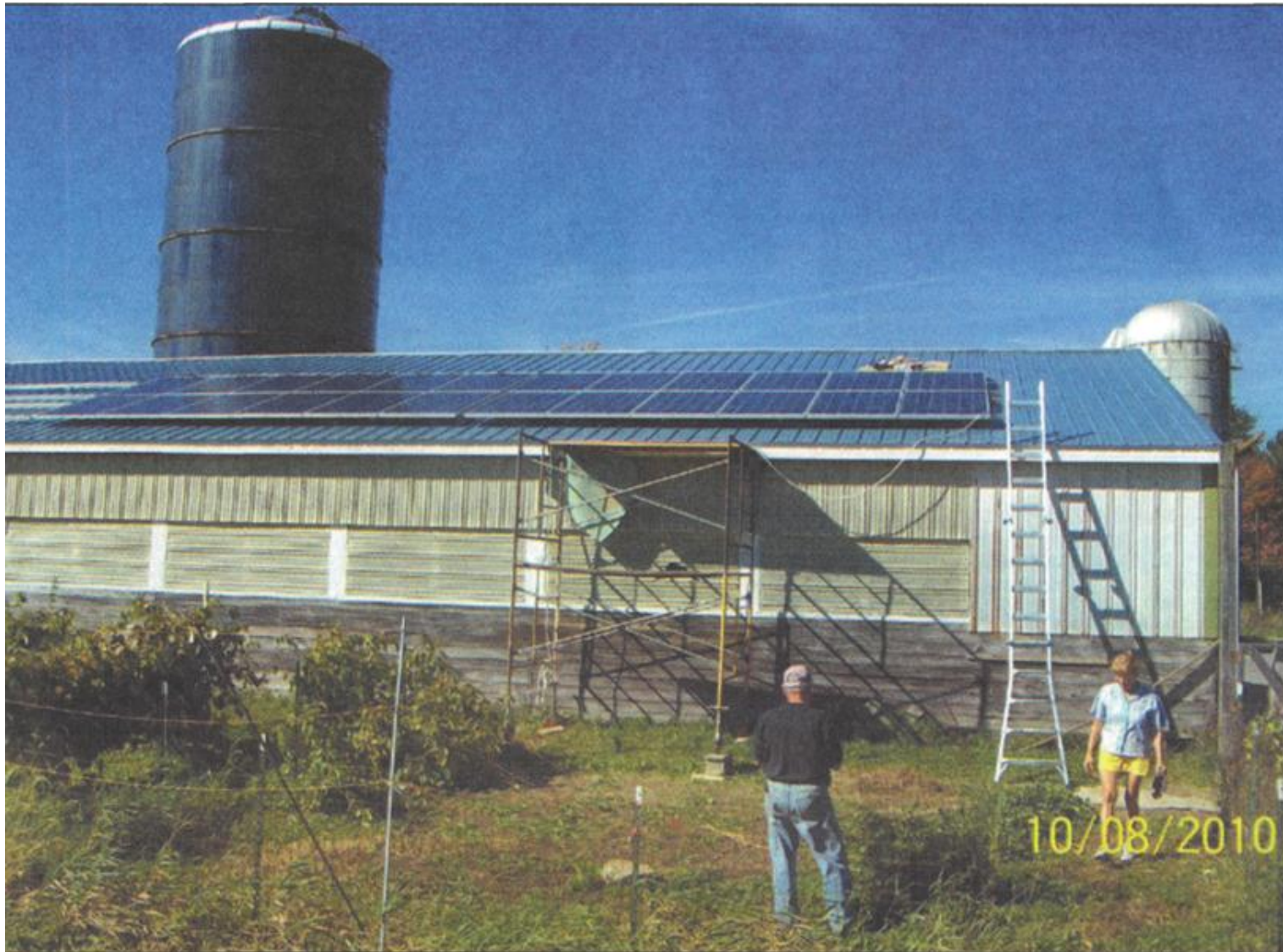
The 10 kw system at Lee and Carol Weber's Blue Roof Farm is mounted on the roof of a barn.
