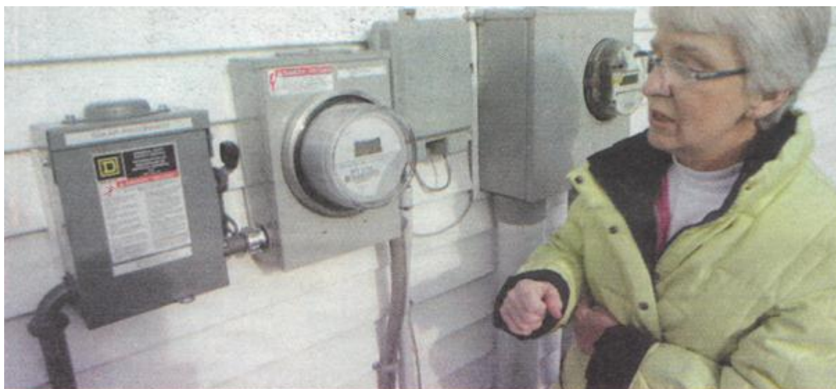
At left, Anita Shaw checks the meters outside her house. Electricity from a power company is used when needed. But when the panels produce excess electricity, the power company takes it and pays for it.
